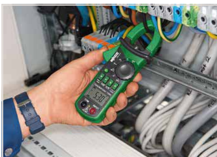
Voltage testing in switchgear cabinet
