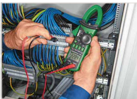
Current measurement in a switchgear cabinet
